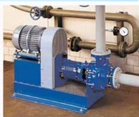
Hidrostat process pump installation.
