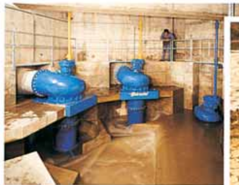
Large sewage lift station equipped with the famous "Prerostal"® flow regulating system
