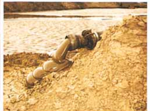
Sludge handling with hydraulically driven mobile Hidrostal pump.
