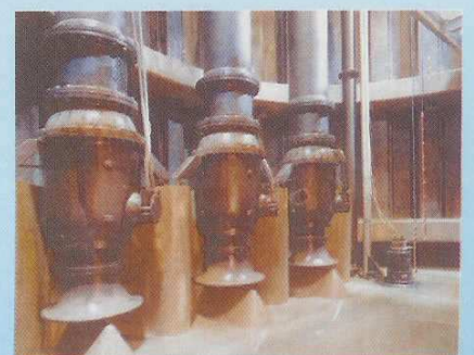
Suspended Wet Well Pumps
